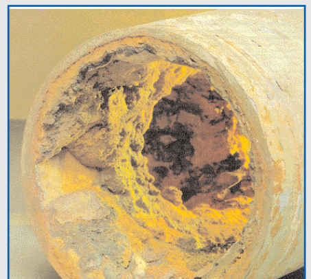
Limestone: it damages pipes and accelerates corrosion.
